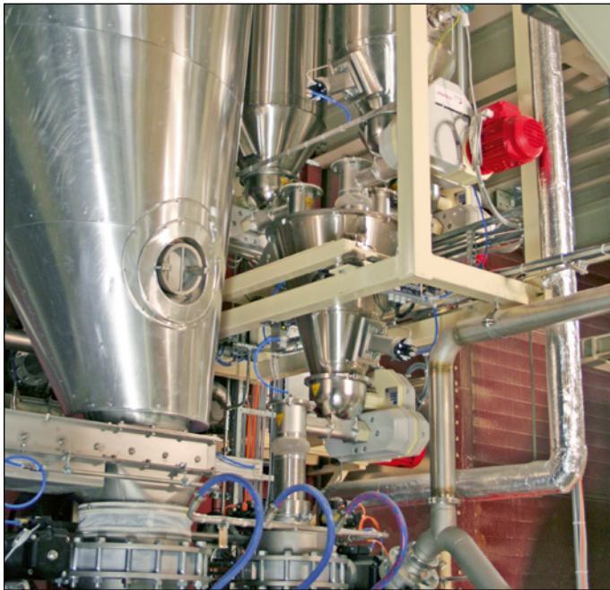
Coperion K-Tron feeders in a pet food coating process
