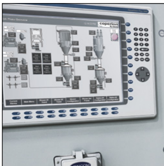
Custom PLC controls
