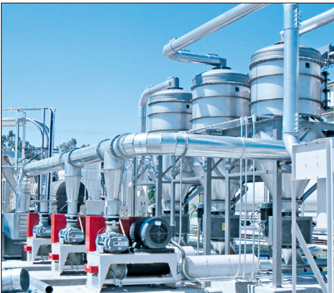
Multi ingredient silo unloading
