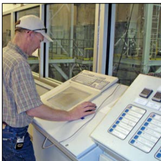
Custom PLC controls
