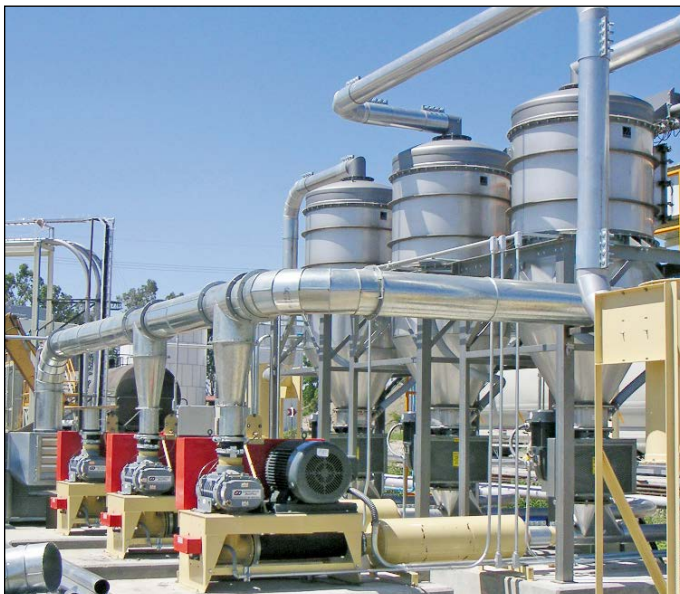
Multi ingredient silo unloading
