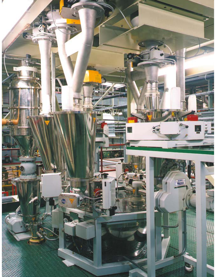
Modular volumetric and loss-in-weight feeders integrated with a gravimetric blending system and pneumatic receivers in a plastics extrusion process
