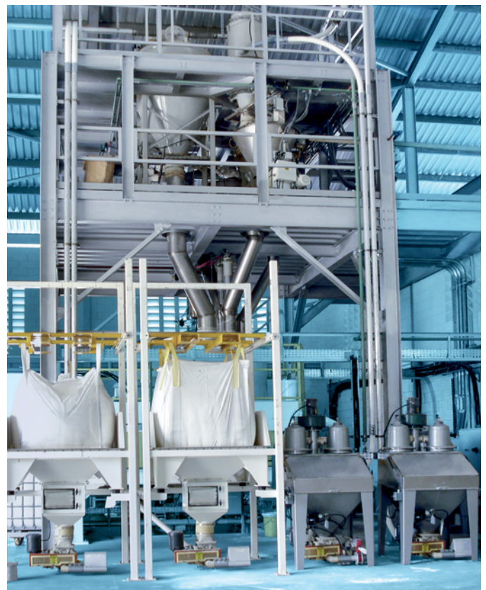
› PVC COMPOUNDING SYSTEM - COMPLETE SYSTEM AND CONTROLS DESIGNED BY COPERION K-TRON IN FULL COOPERATION WITH CUSTOMER TO ENSURE A CONSISTENT AND RELIABLE END PRODUCT.
