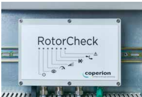
RotorCheck electronics installed in a control cabinet
