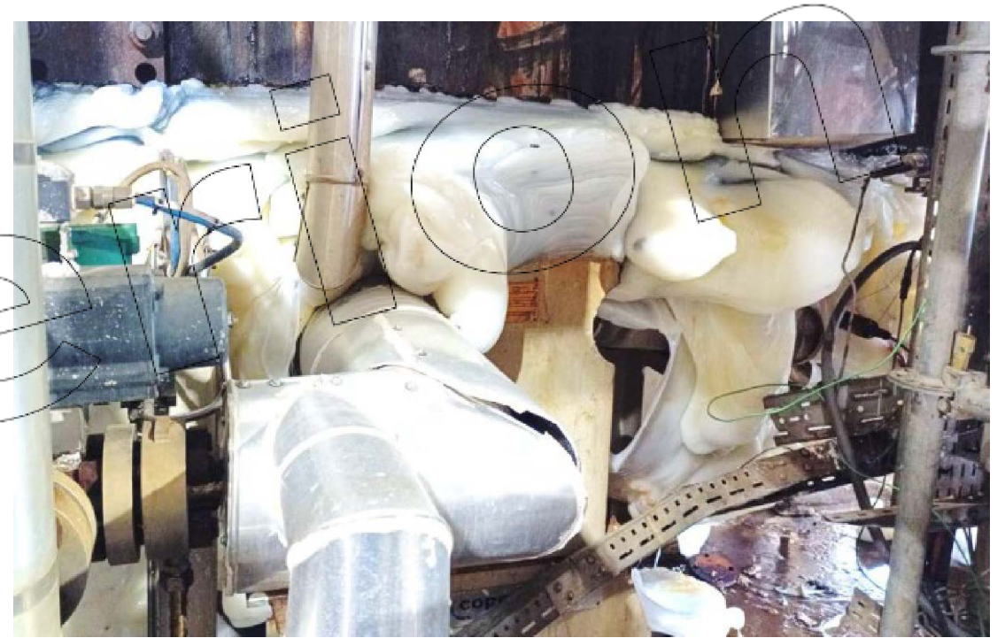
Leaks due to improper house keeping!
